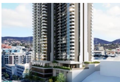
50 Quay Street – a landmark Build to Rent Residential project. Construction is still in progress.
